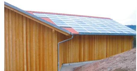
Photovoltaic system on the roof
