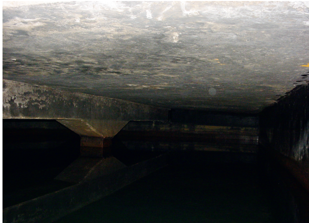
Heavily damaged tank
