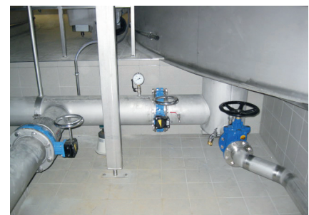
Bottom drain outlet
