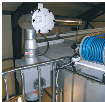
Overflow and air filter system
