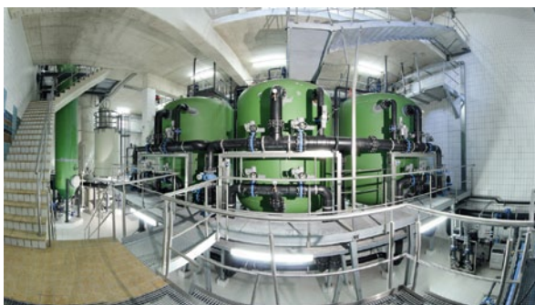
Fig. 3. RDC reactor (left) with filter system (centre).
